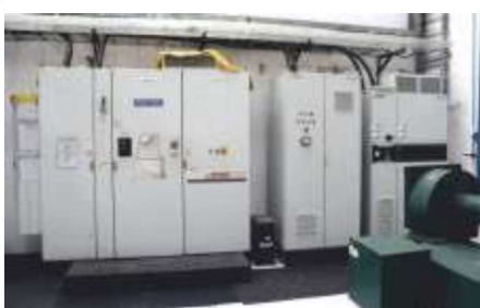
Standby Electric Drive
