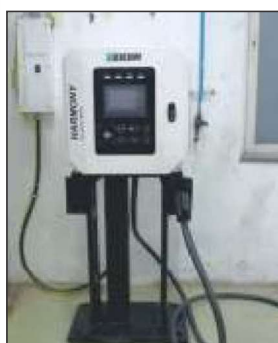
High Voltage Battery Charger
