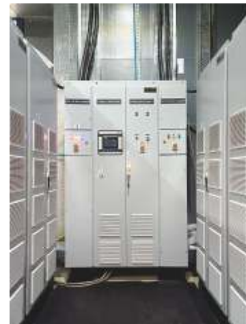
600 kW DC Power Source
